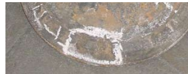
Figure 08: “Cobble stone corrosion” appearance of valve spindle failure through high-temperature corrosion (MC60 Standard-type)
