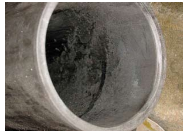
Figure 04a: Breakage of the valve guide during valve spindle disassembling
